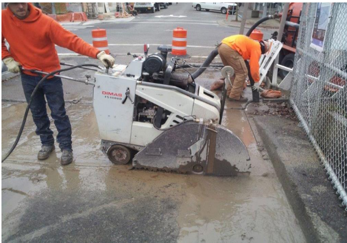
Typical slurry build-up on job using existing technology.
